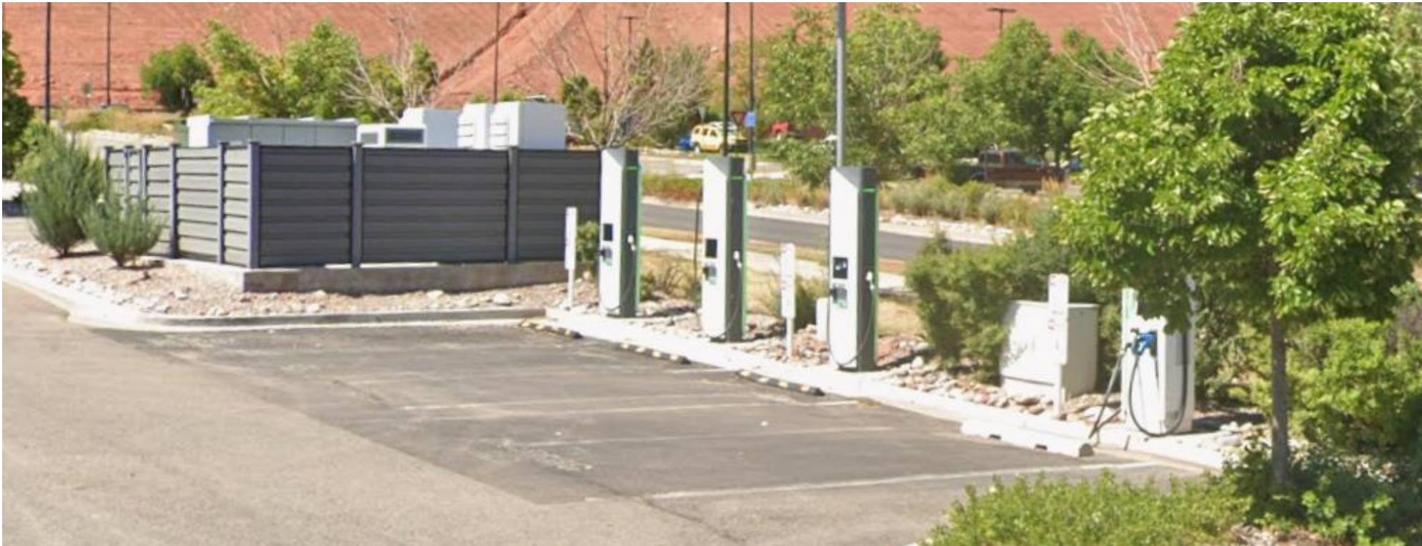
Electrify America Charging Station, Glenwood Meadows
