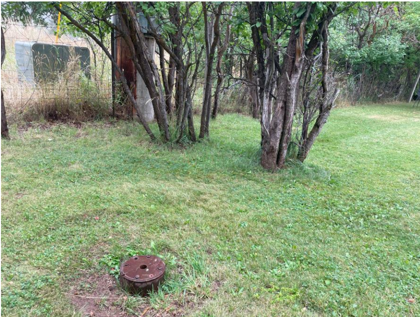
Well, capped. Electrical connection in the background for a water pump.
