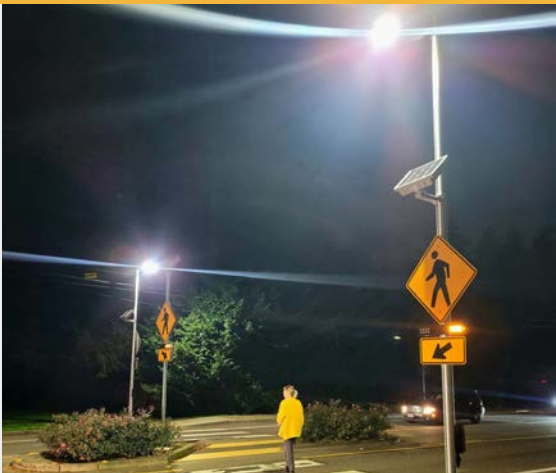
Figure 23. Roadway Lighting (Source: Western Systems)
