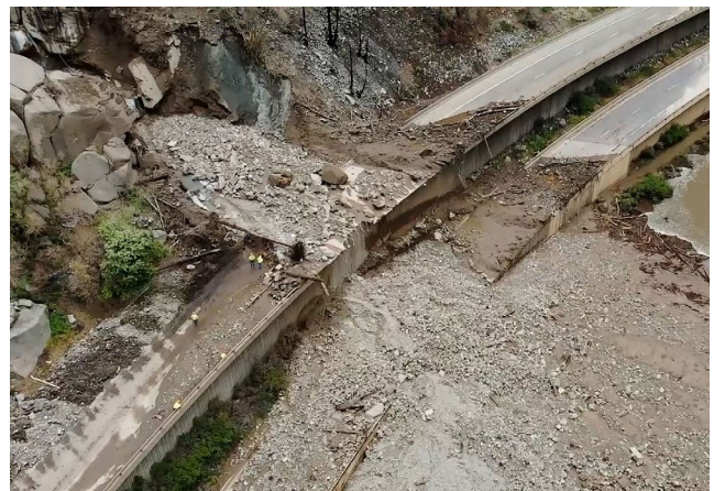
Mudslide on I-70 (Glenwood Canyon) in 2021
