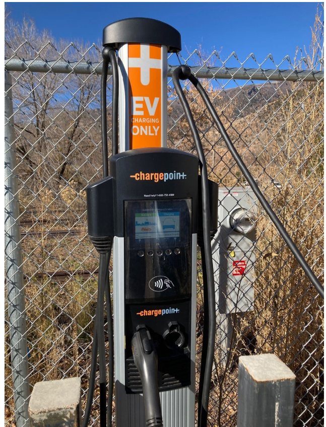
Electric Vehicle Charging Station
