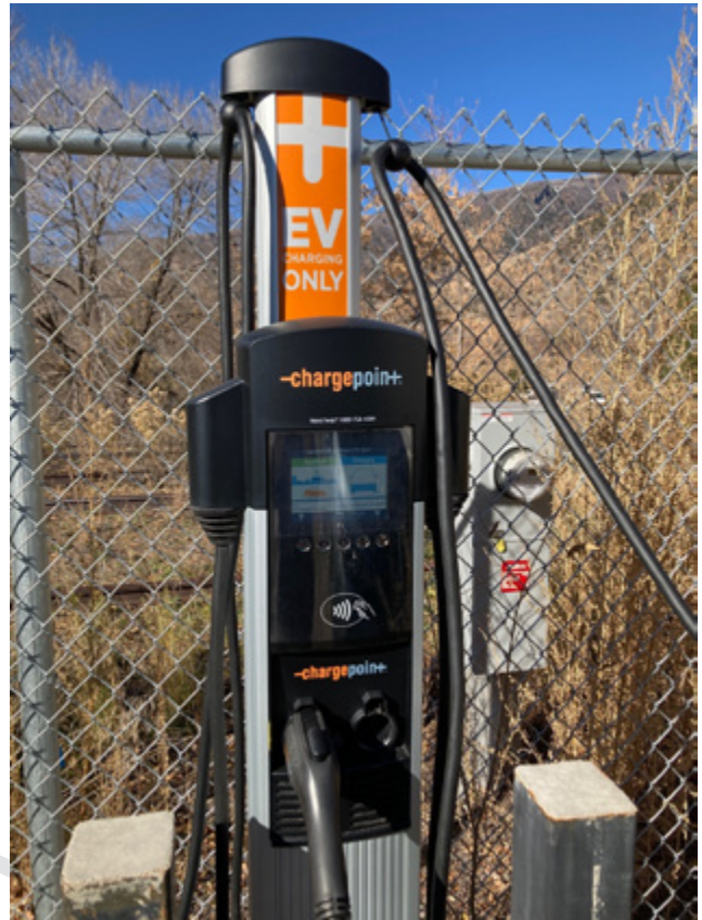
Electric Vehicle Charging Station
