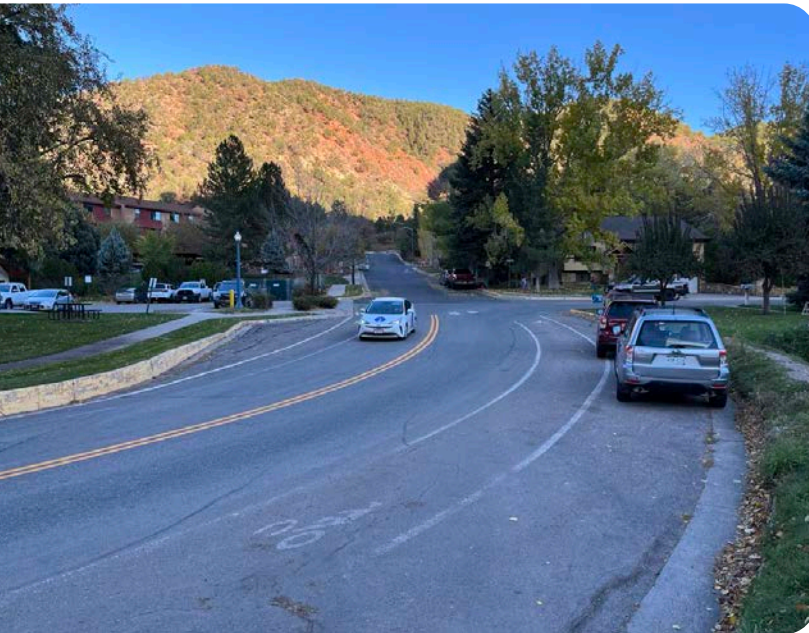
Existing inverted crown and earthen berm near 21st Street where a storm event resulted in a mud slide in the 1970s.
