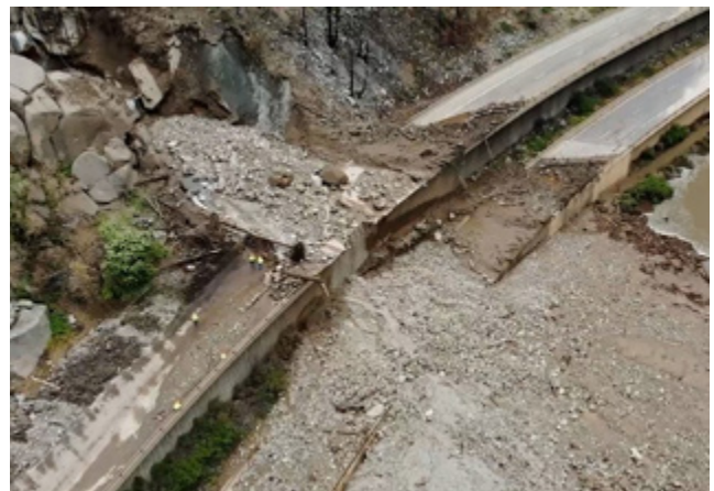
Mudslide on I-70 (Glenwood Canyon) in 2021
