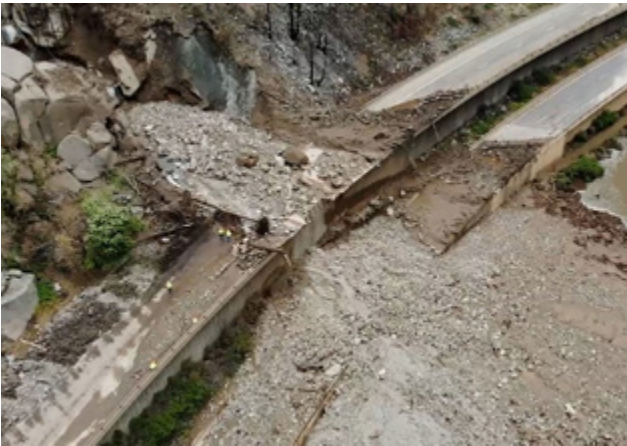
Mudslide on I-70 (Glenwood Canyon) in 2021
