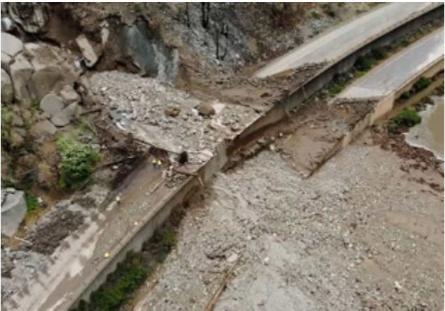
Mudslide on I-70 (Glenwood Canyon) in 2021
