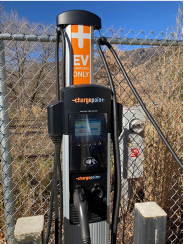
Electric Vehicle Charging Station
