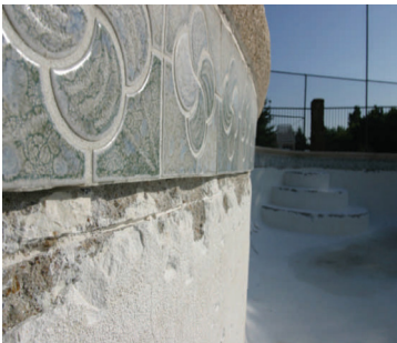
Saw-cut and chip below tile
