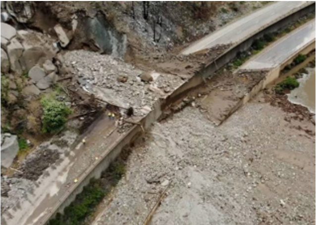
Mudslide on I-70 (Glenwood Canyon) in 2021
