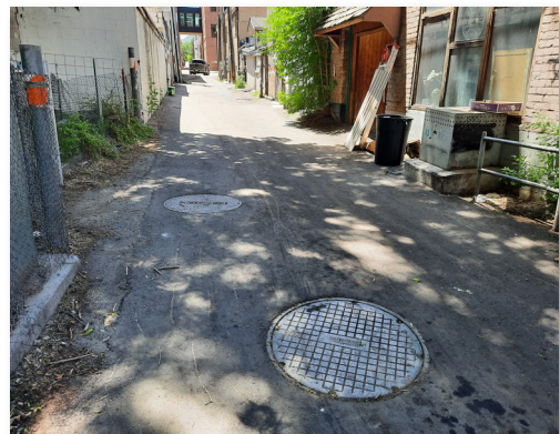
Block 44 electric manholes
