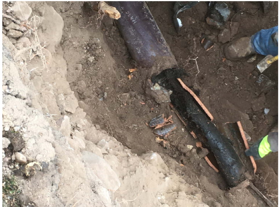
Collapsed Sewer Line with Root Intrusion
