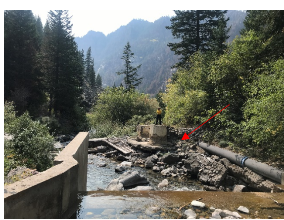
Concrete loose materials.
