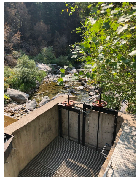
Waterman gates and headwheels, and derrick mount would need to be changed out for plate to sit on vault.
