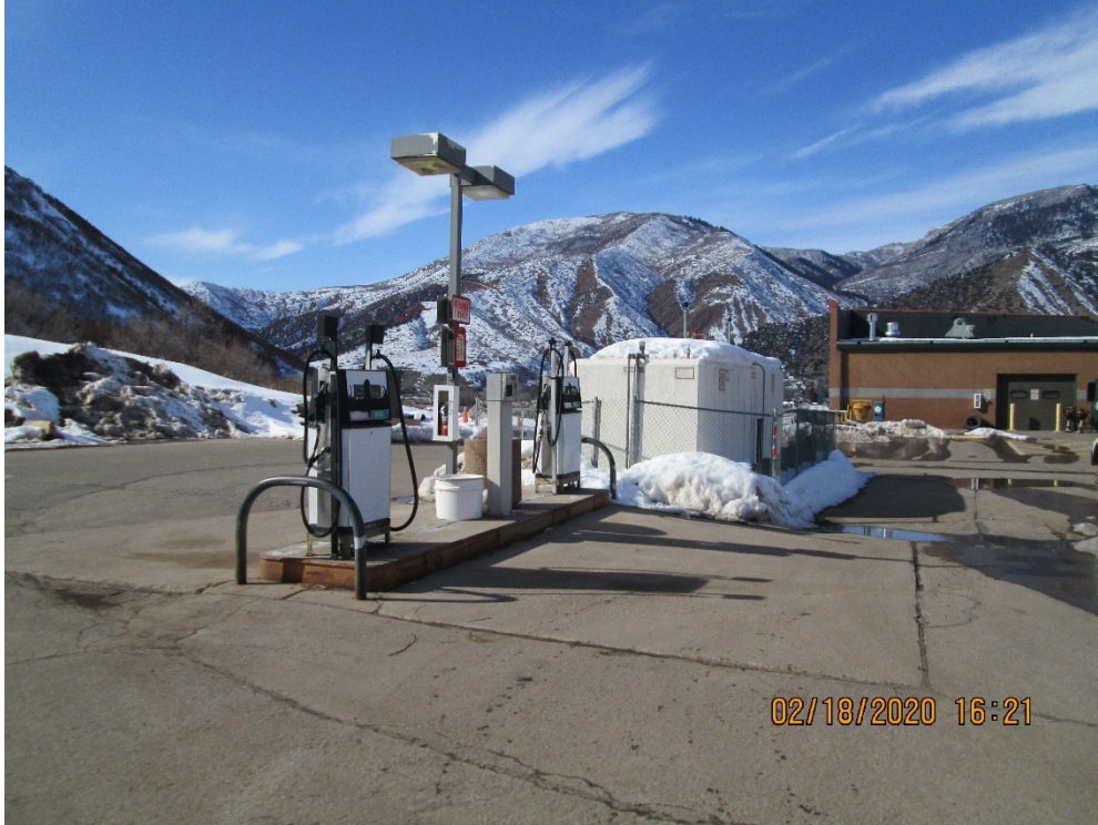
Existing MOC gasoline pumps and above ground fuel storage.
