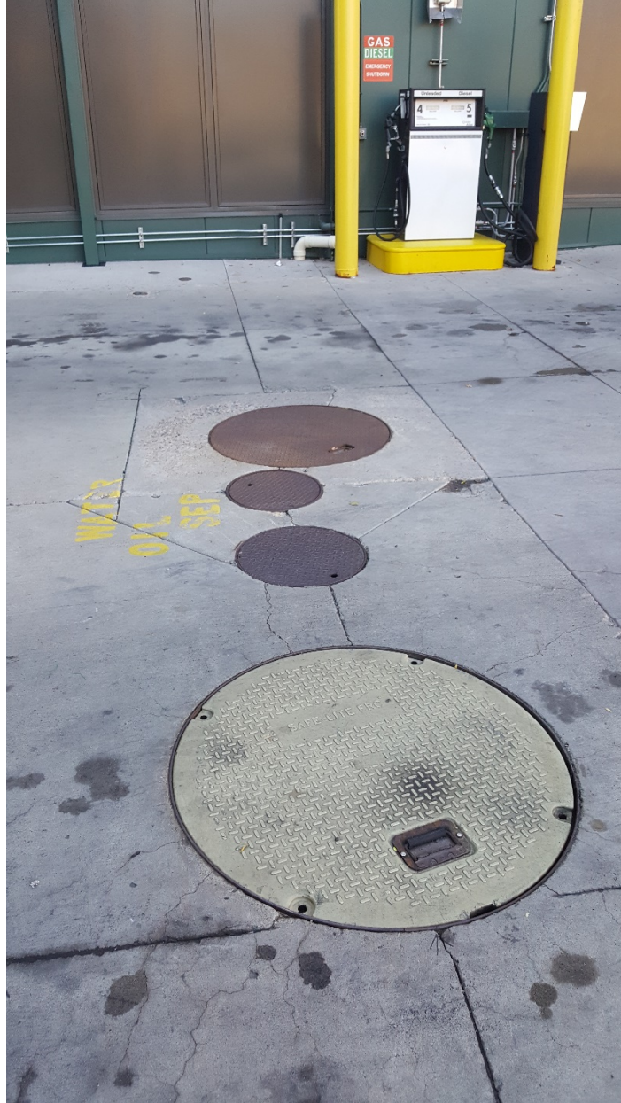
Photo 9-Oil water separator pit with controls, looking from the north
