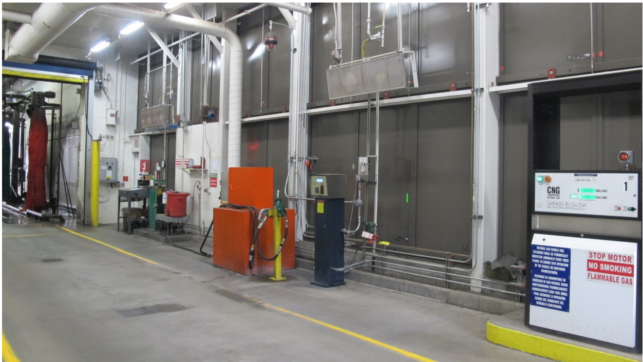
Photo 11-Fueling and wash bay
