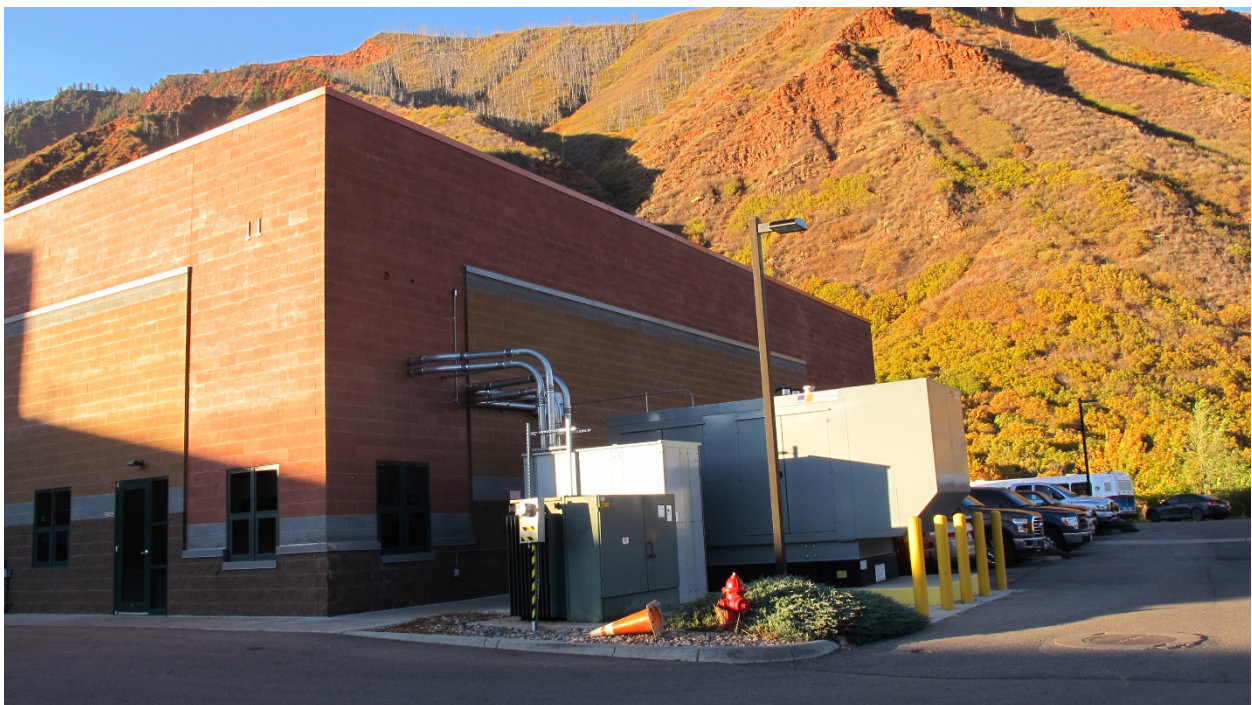
Photo 6-Utility equipment pad on north end of existing GMF building
